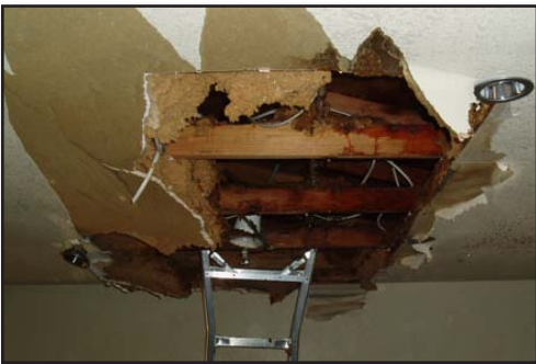
Figure 23-3 Gypsum becomes heavy when wet and ceilings may collapse without warning
