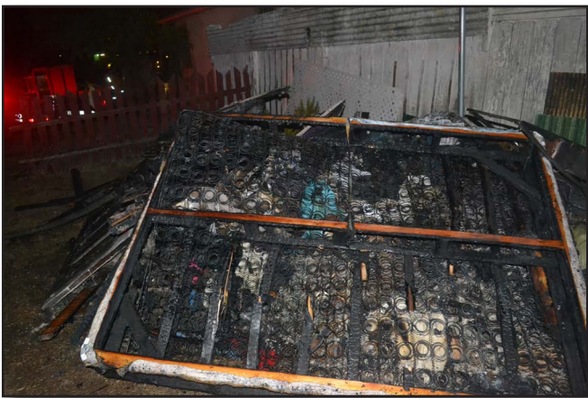
Figure 23-23 The debris pile should be placed on the property in a location that will not create any further damage to the structure should it re-ignite. Continuous wetting of the layers of the debris pile is often necessary to prevent a rekindle.
