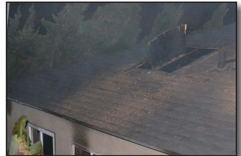
Figure 23-27 Ventilation holes should be covered with visqueen prior to turning the structure back over to the homeowner.
