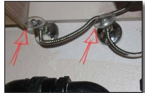
Figure 23-10 Localized water shut-of valve
