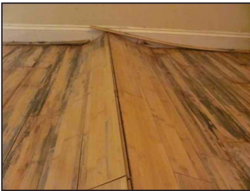
Figure 23-2 Water damage to wooden floors
