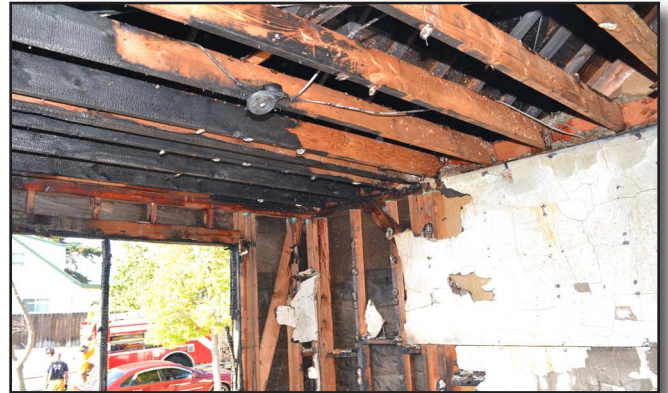
Figure 23-20 An attic fire necessitates the removal of all ceiling and insulation material. Blown in insulation is especially problematic in regards to rekindle and must be removed entirely, resulting in a lengthy overhaul process.
