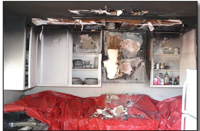
Figure 23-14 Salvage cover used to protect the lower cabinets and counter tops prior to overhaul of the ceiling.
